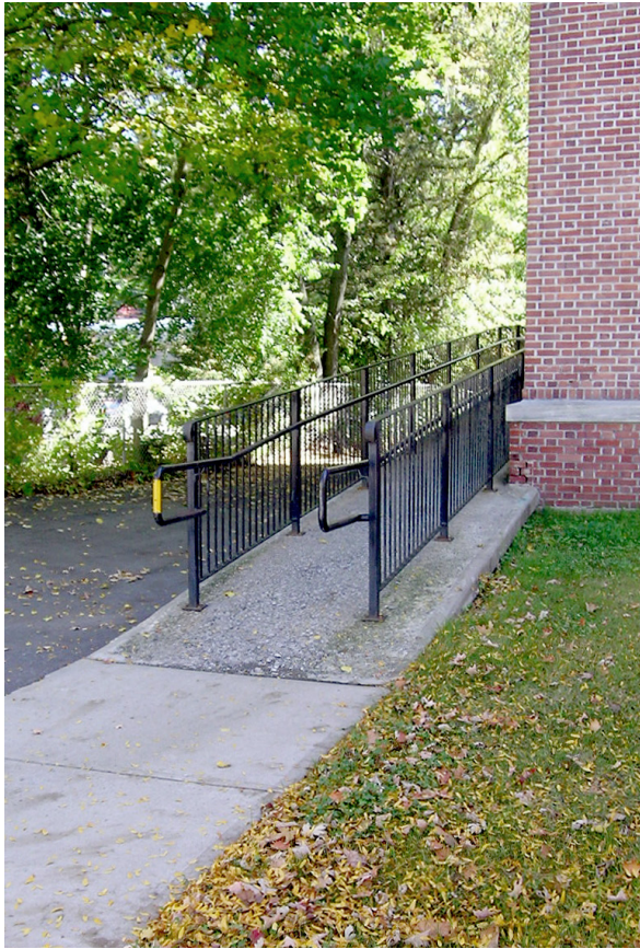
(Left) The surface of the handicap accessible ramp is badly worn from roof run off, and mortar has washed out from the mortar joints above the area where the ramp intersects the west wall. [JGWA 2014]
