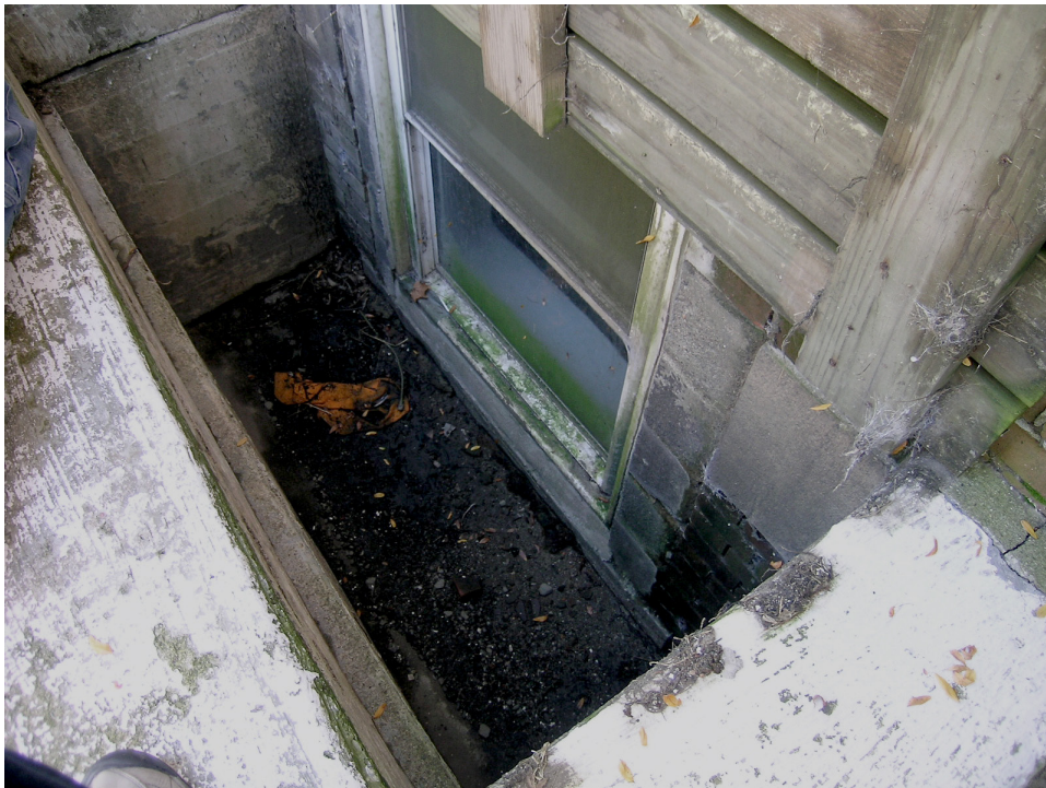
(Below) The original masonry opening of the northwest window well has been reduced with concrete block, and the contemporary replacement window is covered in biological growth. All window wells are damp. At the right, a large mortar patch was used to fill the gap where the top of the window well has frost jacked away from the wall. [JGWA 2014]
