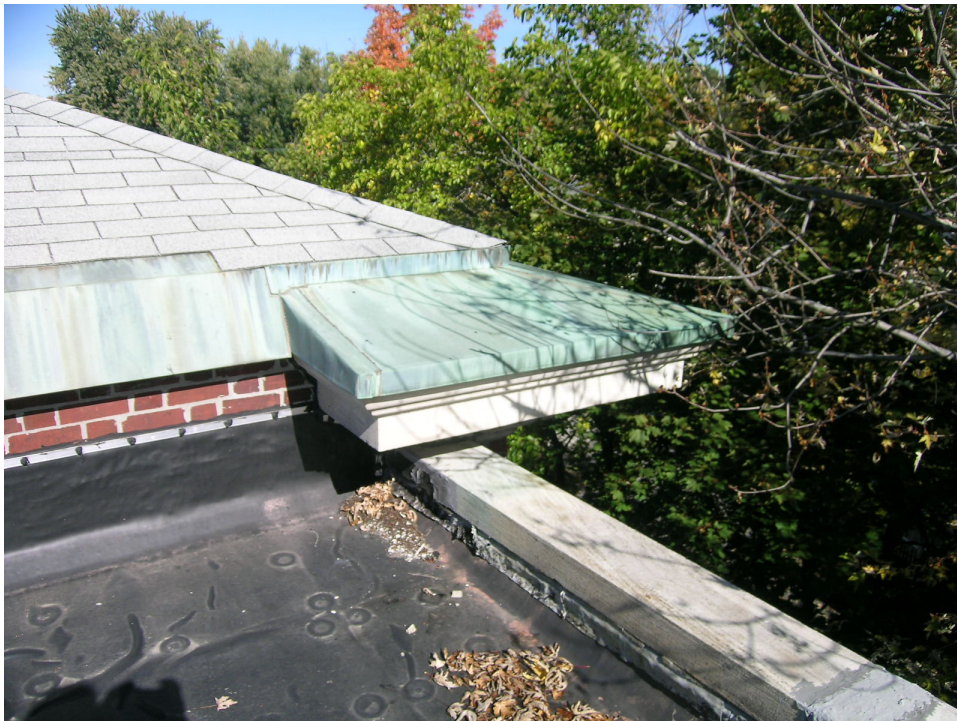
(Below) The step in the roof slope indicates the location of historic built-in gutters, which have been covered over with copper flashing. [JGWA 2014]
