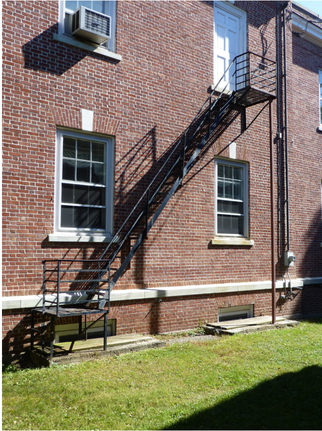
(Left) Electrical service entrance, metal fire escape, and second floor emergency exit in a historic window opening at the south elevation. [JGWA 2014]
