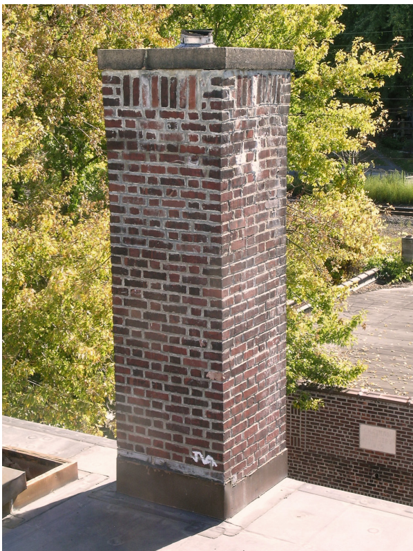
The chimney is no longer plumb, and leans slightly. Numerous joints have been repointed with inappropriate mortar or sealant. Cracked brick joints and units contribute to water infiltration and damage to the spaces below. [JGWA 2014]
