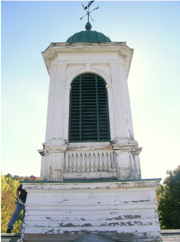
Cupola paint is badly worn and there are numerous areas of missing or inappropriate wood trim replacement. Metal roofing and flashing is poorly detailed. [JGWA 2014]
