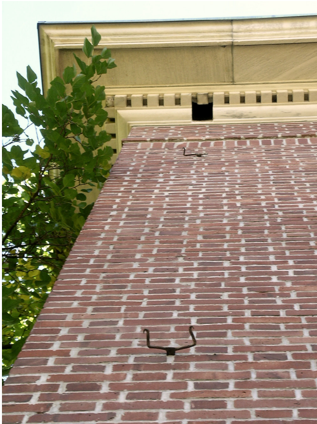
(Left) Former roof leader location and hangers. West elevation shown. Also note the proximity of mature trees on the north elevation. [JGWA 2014]
